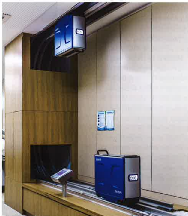
Telelift systems fit seamlessly into the hospital design, and include features such as antimicrobial coating to meet sterilisation standards.
